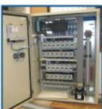
Starter Panels for Conveyors
