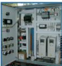
Pump Control Panels
