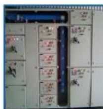
PLC Panels for Pneumatic Control Housing
