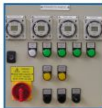
Boiler Control Panels
