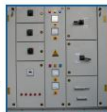
Starter Control Panels
