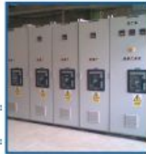
PCC Control Panels
