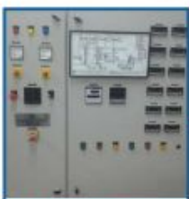
AC Drive Panels
