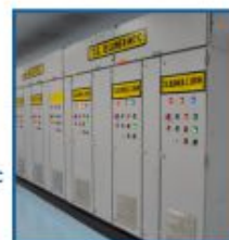
Variable Frequency Drive Panels
