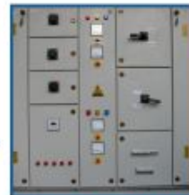
Starter Control Panels
