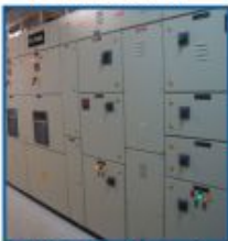
AMF Control Panels
