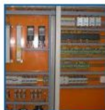
DC Drive Control Panels
