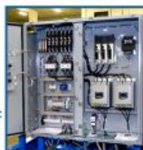
Drive Panels for Pumps
