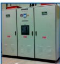
APFC Capacitor Panel
